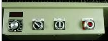
System control panel.
